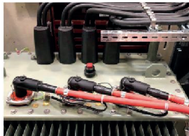
Transformator z K180AR-3/J i K200LR
