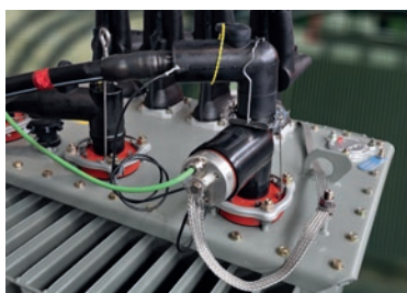
Transformator z K180AR-1/J, K200LR i adapterem KAA4-OS
